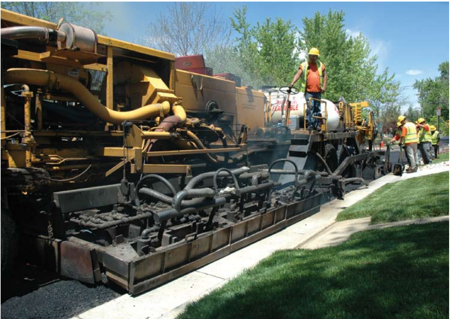
Heating, scarifying, applying rejuvenating agent and applying new overlay is done in a one-pass process with the proprietary equipment Cutler uses. The process delivers a high-quality road with fewer disruptions at a lower cost than conventional mill and overlay roads.
