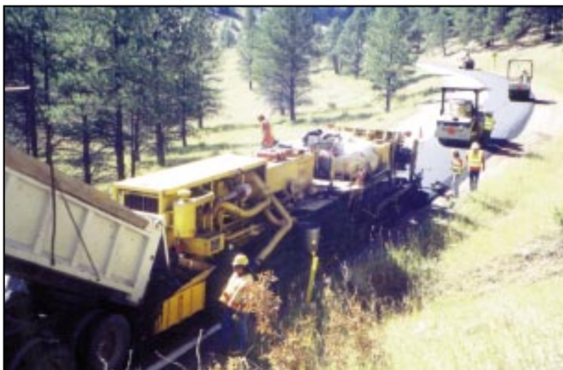
The machine travels quickly and lane closures are minimized. All reclaimed material is used on the spot without hauling and truck traffic is eliminated.
