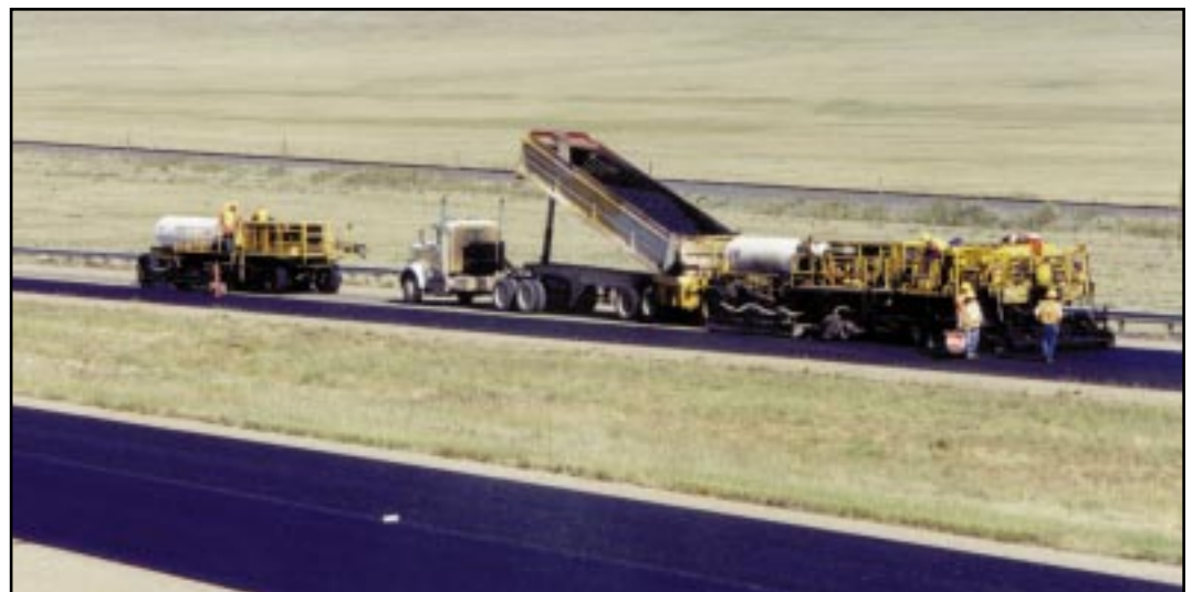
Cutler's hot-in-place (HIP) recycling process, called Repaving, provides a virgin hot mix asphalt (HMA) driving surface bonded to a leveling or base course incorporating the recycled former road surface, shown here on I-25 in Las Vegas, New Mexico.
