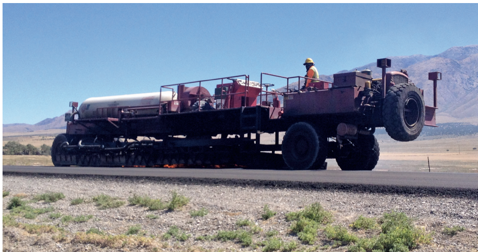
Propane heaters were employed to prepare the existing degraded surface for recycling.
