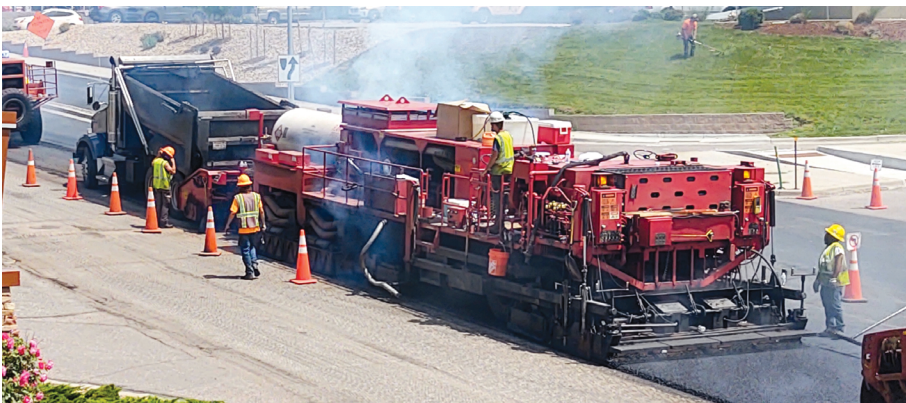
A paving train with pre-heater followed by repaver on County Line Road in Littleton, Colo. CREDIT: TODD GONSER
