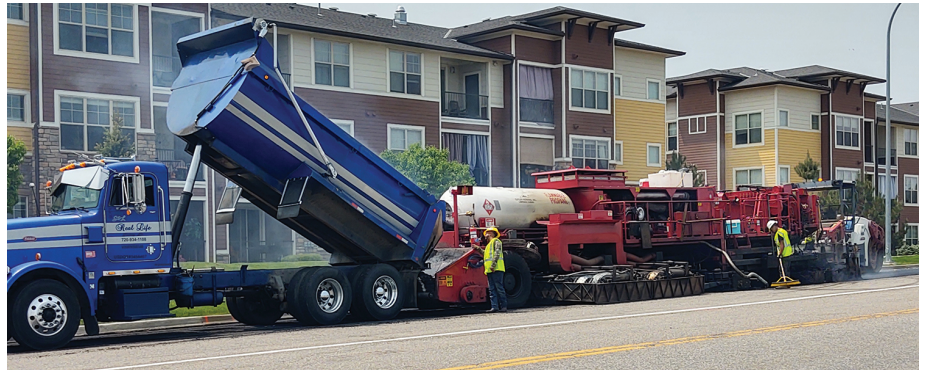
A crew in Littleton, Colo. operates a paving train in front of an apartment building. CREDIT: TODD GONSER
