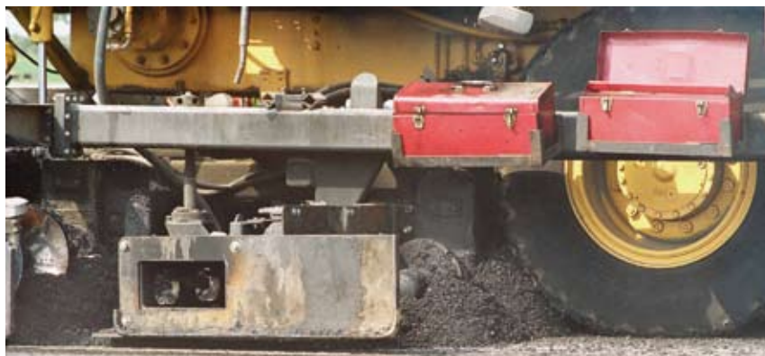
The top photo shows the one-pass asphalt recycling method in action. The middle photo shows the recycling agent being applied and mixed, while the bottom photo shows the recycling screed laying the recycled mix.
