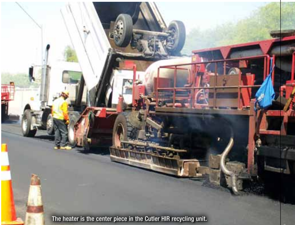
Kansas-based Cutler Repaving's hot recycling train is led by a pavement preheater. The mobile recycling unit comes next, and it is fed hot mix asphalt for the overlay. The recycling unit heats, scarifies, adds a recycling agent, remixes the material, spreads it and lays the overlay on top.
