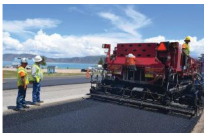
The recycling screed gathers and lays the recycled material in advance of the main paving screed.
