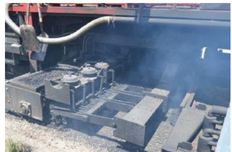
Carbide-tipped teeth cut the heated, softened pavement in a level plane without breaking apart the individual aggregates in the existing pavement.
