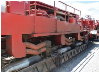
The existing pavement is initially softened with the first application of heat applied by the preheater conveying vehicle in advance of the main repaver.
