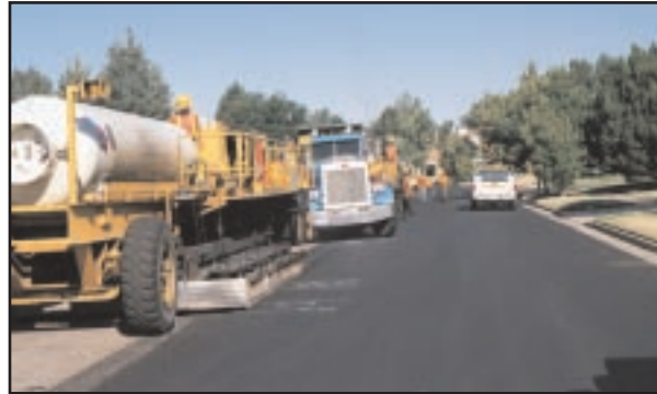
Rebeated edge of repaved lane results in high density seam between lanes
