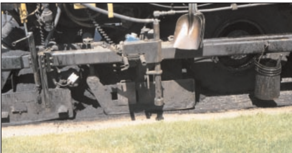
Reclaimed asphalt is reapplied and distributed with a screed as a 1 inch leveling course
