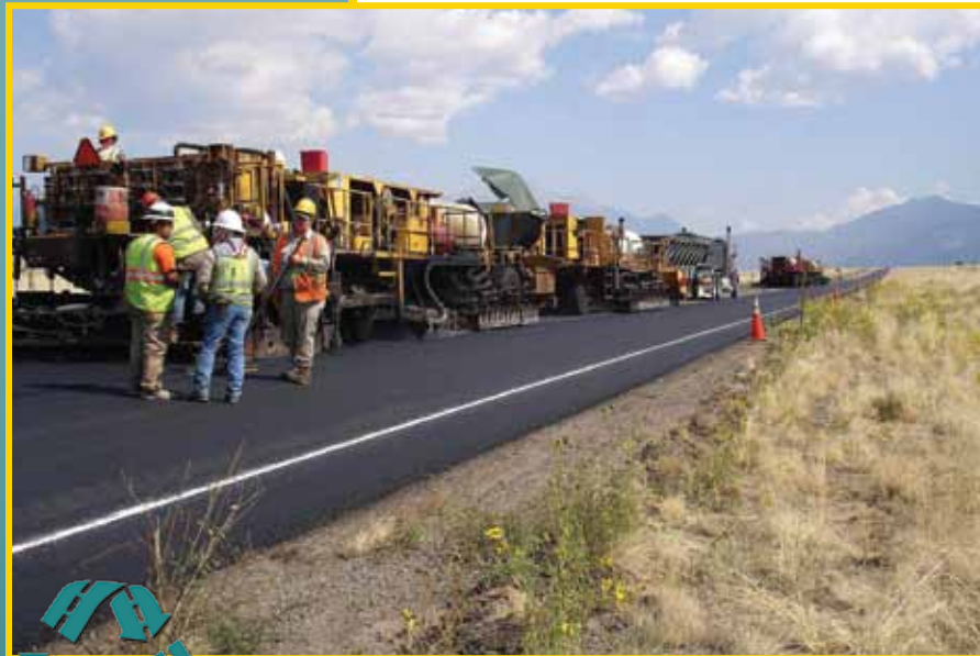
Hot in-place recycling (HIR) train on Colorado S.H. 150 included, from left, repaver, preheater, virgin HMA haul unit for surface course, and auxiliary preheater.
