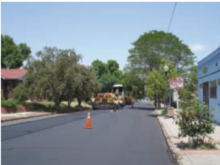
Denver enhances the sustainability of its repaving program by using up to 40 percent reclaimed asphalt pavement in the hot-mix wearing course.
