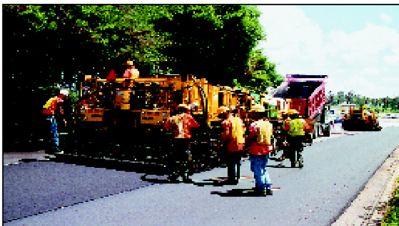
Main Repaver unit beats asphalt to 300 deg F, scarifies to a depth of 1 inch and mixes scarified material with rejuvenator; then reapplies reclaimed asphalt pavement and places additional lift of virgin mix on top.
