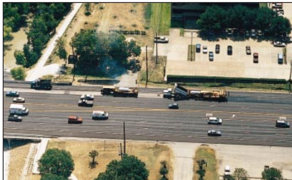
J. A. (Tony) Yrigoyen, Design Engineer for the Texas Department of Transportation West Area Office, relied on one-pass, hot in-place recycling (HIR) for successful repaving of seven-lane State Highway 6 in suburban Houston
